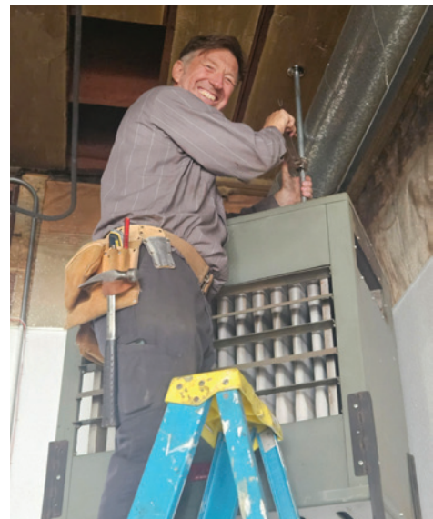
At top: Old labels and nails hang on the old rafters, perhaps as part of a display or sale in the building's previous life. Above: Owner Larry Guenther works on the building's heating system.
